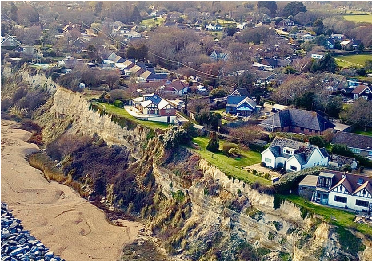
Figure 4.2: The publication of practical advice for home-owners can raise awareness amongst those living within the Coastal Buffer Zone thereby helping to encourage good practice in property management and maintenance and avoiding acceleration of cliff instability. Photo: Isobel Horsley.
